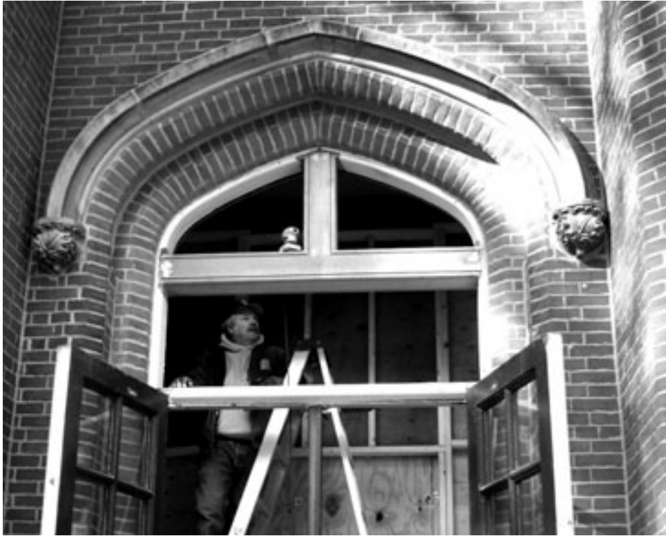
Charles Groshong fits transom built by Historic Restorations into Old Main at Franklin & Marshall College.
